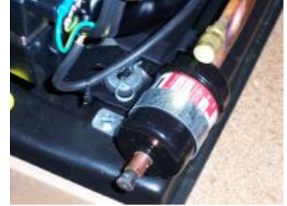
A strap and single screw hold filter/dryer to compressor base.
