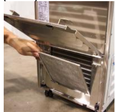
Inspect the condenser coil filter. If dirty, wash in the sink and allow to dry before replacing.
