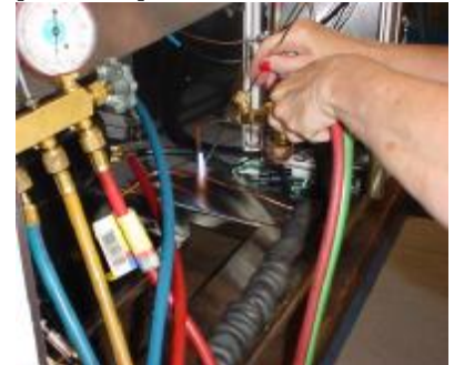
When resealing the system, use a continuous Nitrogen charge to keep contaminants out.
