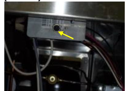
Controller is mounted above left side vented access panel opening.
