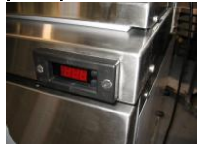
Remote Temperature Display installed with new heavy duty protective bezel.
