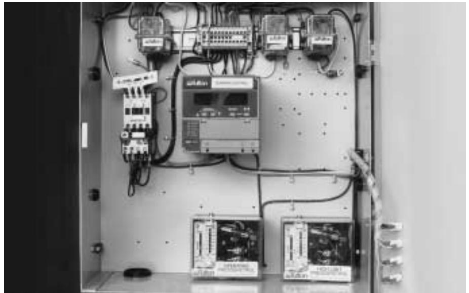
60 HP – 7800 flame safeguard control
