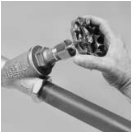
Blow Down Boiler Daily. Shown is the blow down "Y" valve.
