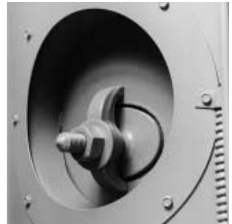
Inspect hand holes for scale or sludge buildup.
