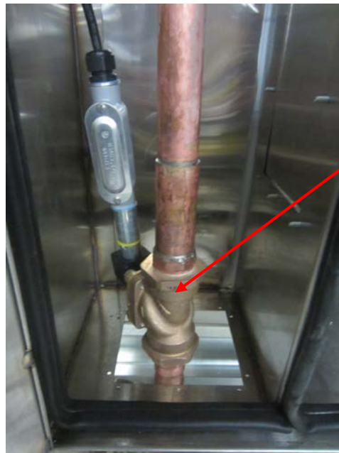
Figure 4-50-1 Water Solenoid Valve
