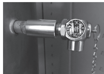
The pressure relief valve must face downward.
