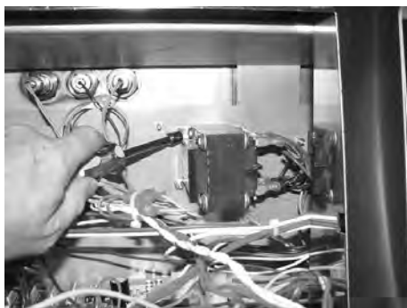
Express Filter Transformer
