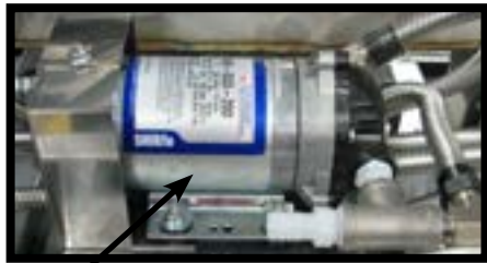
Located behind motor
