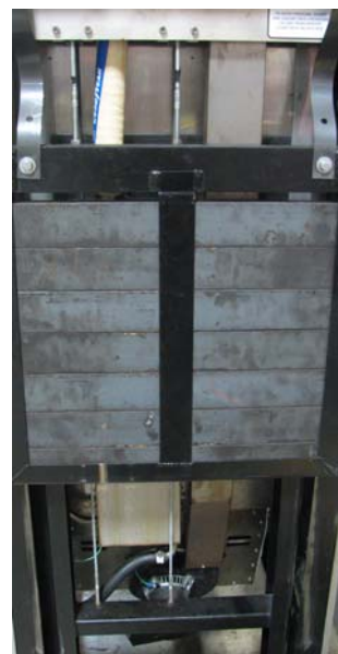
View of the counter-weights with cover removed
