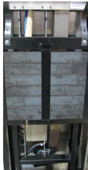
View of the counter-weights with cover removed
