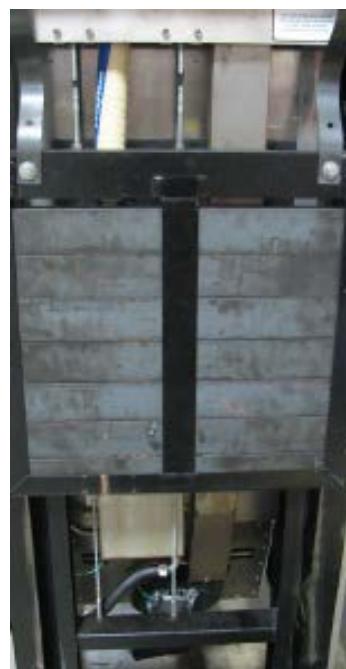
View of the counter-weights with cover removed
