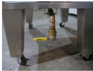
Valve in closed position
