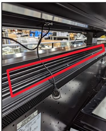
Fig. 8 Accessing power supplies for shelf lights
