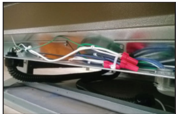
Fig. 7 Raceway electrical wiring
