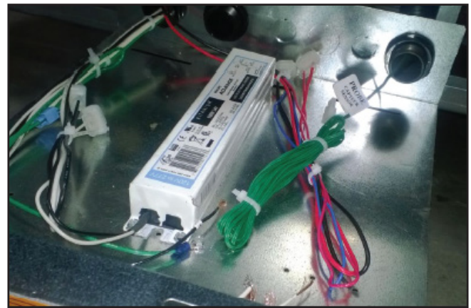
View of power supplies inside case
