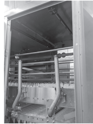
Low Temp Chemical Rinse
