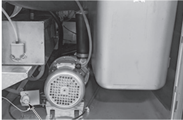
HOT WATER CONNECTION
