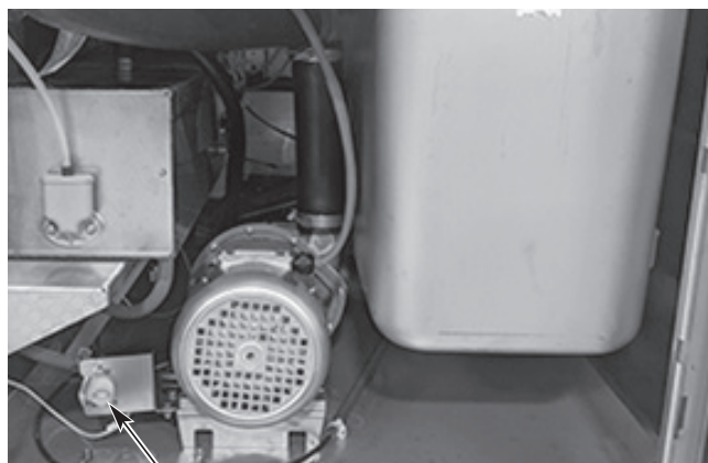
HOT WATER CONNECTION
