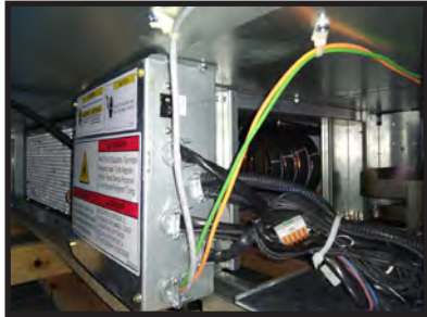
Controller Electrical Box
