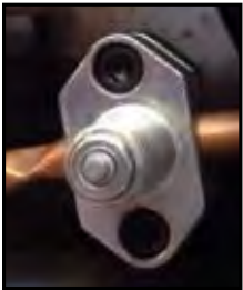
refrigeration line tapping valve
