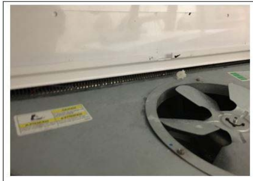
Incorrect – evaporator coil can be seen between back panel and fan plenum
