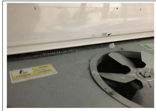
Incorrect – evaporator coil can be seen between back panel and fan plenum
