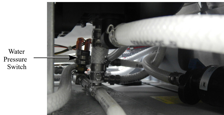
Figure 80. View of Water Pressure Switch
