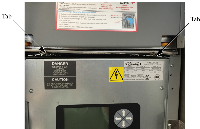
Figure 63. Air Filter Location
