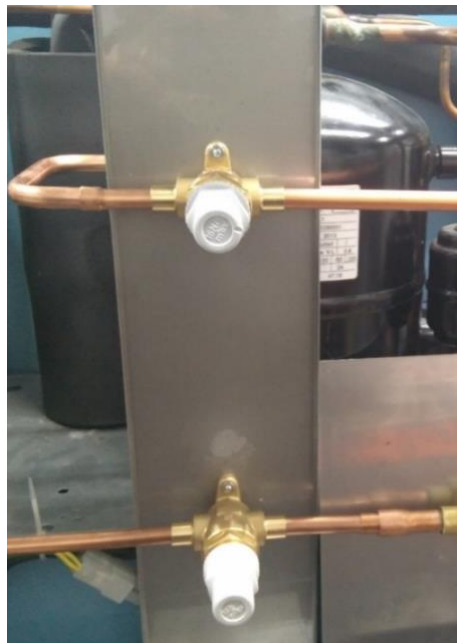
Picture 6: Cut-off valves inside the ice machine
