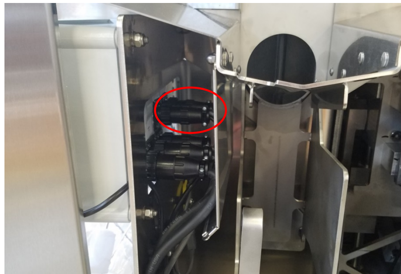
Figure 69. Location of Safety Cables
