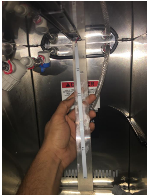
Figure 90: Light Cover removed.
