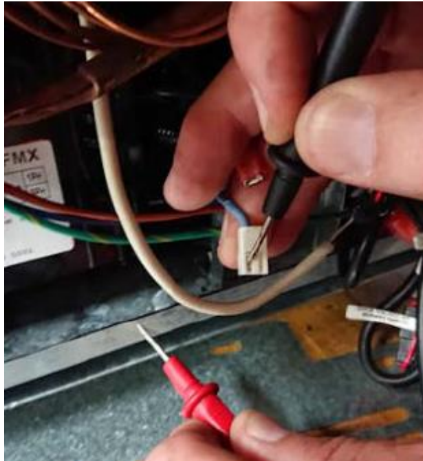
Figure 75: Voltage being probed.
