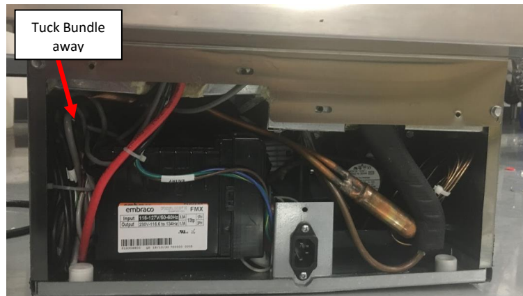
Figure 124: Wire Bundle tucked away.
