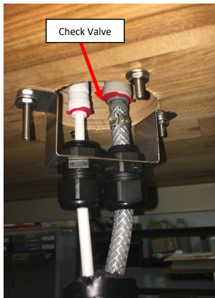
Figure 28a: Check Valve Shown.
