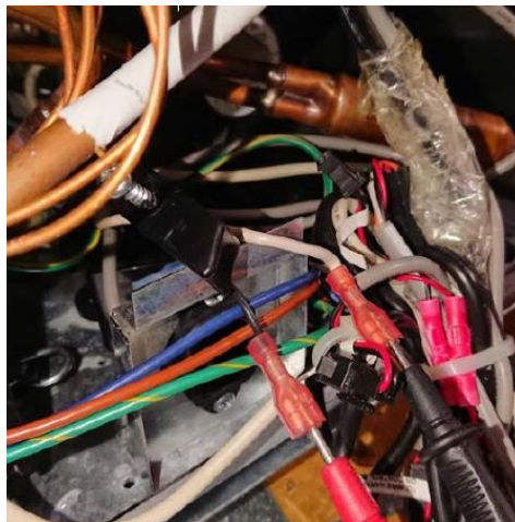
Figure 73: Line Voltage being probed.
