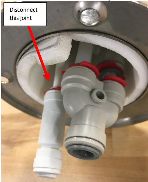
Figure 45a: Check Valve connection Shown.
