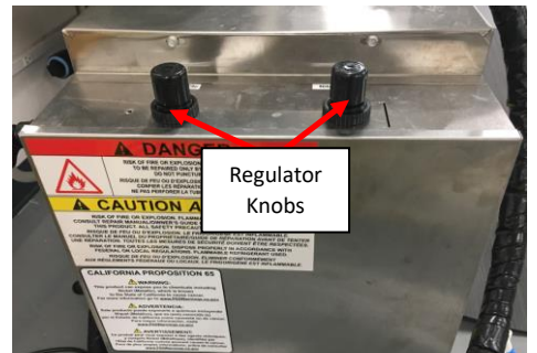
Figure 21c: Pressure Regulator Knobs on the Rear Enclosure.
