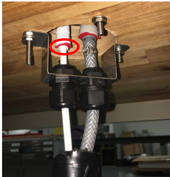
Figure 52: Check Valve Leak Test Location.
