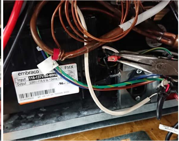
Figure 72b: Power connections shown removed.
