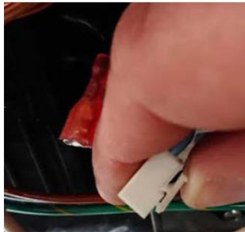
Figure 74a: Line Voltage being probed.
