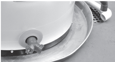
Figure 8 - A suitable drain pan piped to an adequate drain can help protect flooring from leaks and drips.
