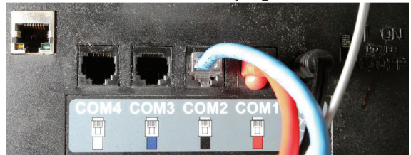
Figure 1: COM ports on the back of the Kitchen Minder are connected to Merco Translators, which are in turn connected to a Merco holding cabinet.
