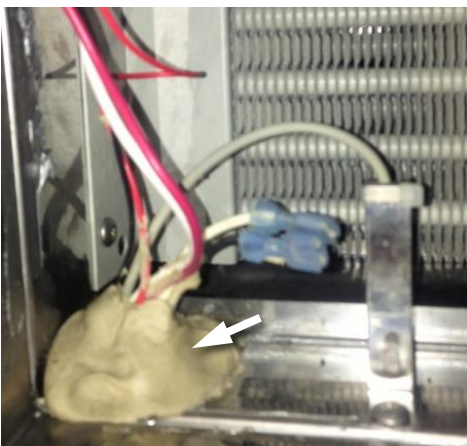
Figure 6-1. Sealing Compound at Wiring Pass-through
