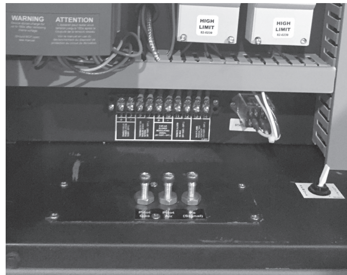
Figure 16 Manometer connections to the test manifold (in control cabinet)
