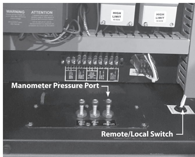
Figure 21 Manometer connections to manifold
