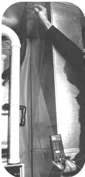
FIGURE 47 TEMPERATURE RISE MEASUREMENT
