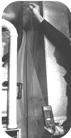
FIGURE 57 TEMPERATURE RISE MEASUREMENT
