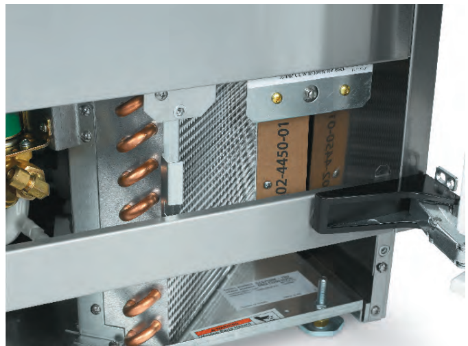
Condenser and Bin Thermostat
