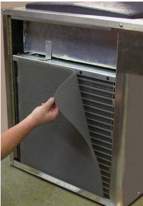
Figure 3-11 F112 Condenser Filter Removal
