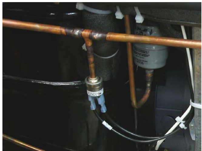
Figure 5-6 High Pressure Cutout
