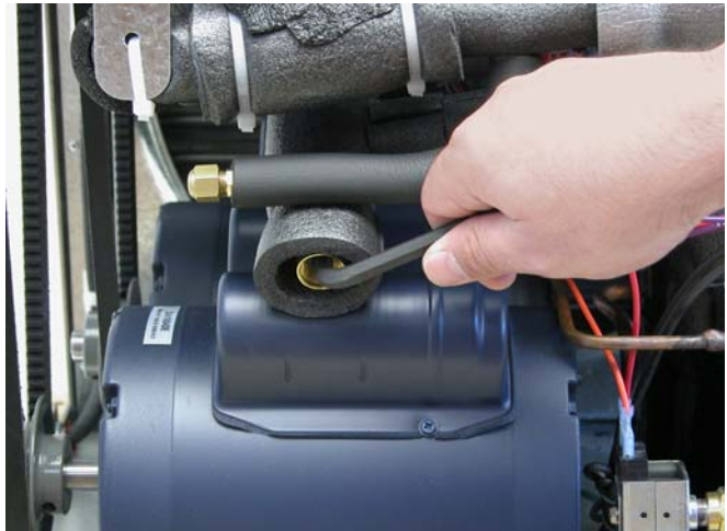
Figure 5-8 Hot Gas Bypass Adjustment
