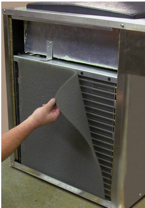
Figure 3-11 F112 Condenser Filter Removal
