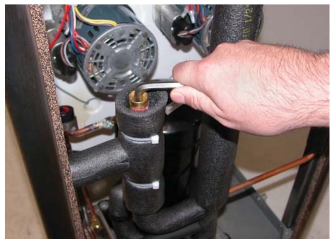
Figure 5-8 Hot Gas Bypass Adjustment
