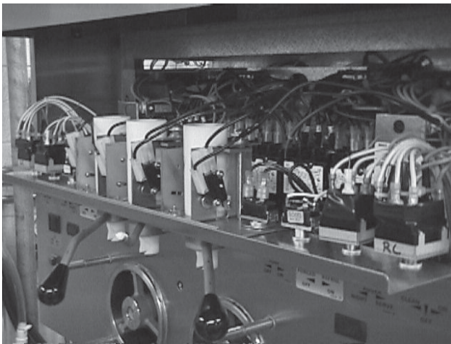
Figure 45. Front Electrical Box
