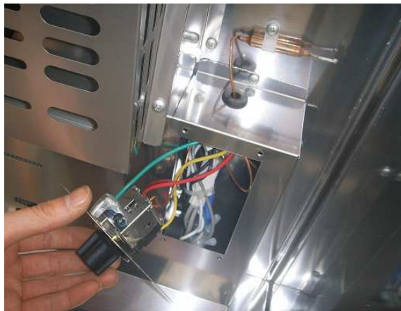
TEMPERATURE CONTROL & EVAPORATOR
