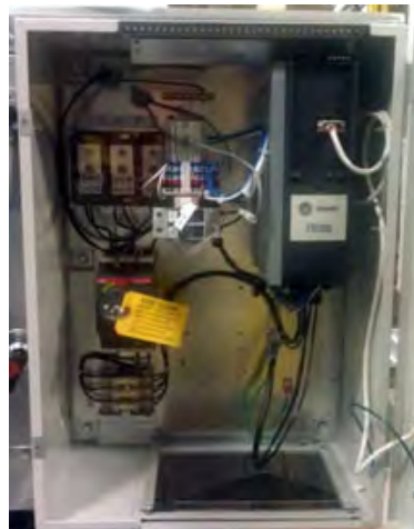
Figure 141. Externally mounted VFD
