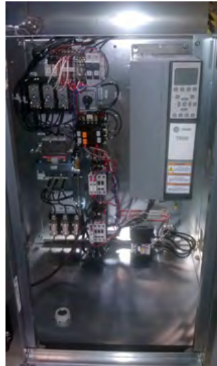
Figure 140. Internally mounted VFD
