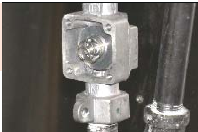
7 New spring/magnet assembly installed
