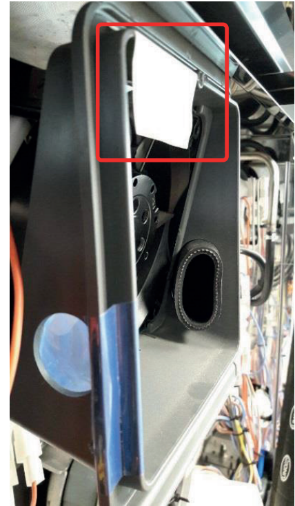
Fan is not running in the right direction
