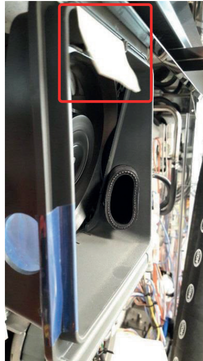
Fan is running in the right direction
